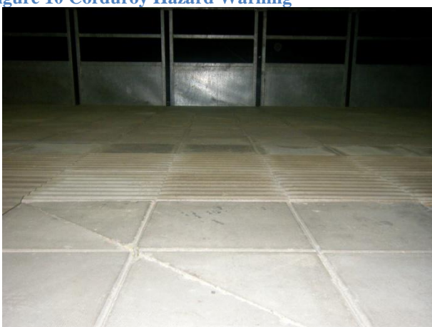
Figure 12 Corduroy Hazard Warning raised 6mm
