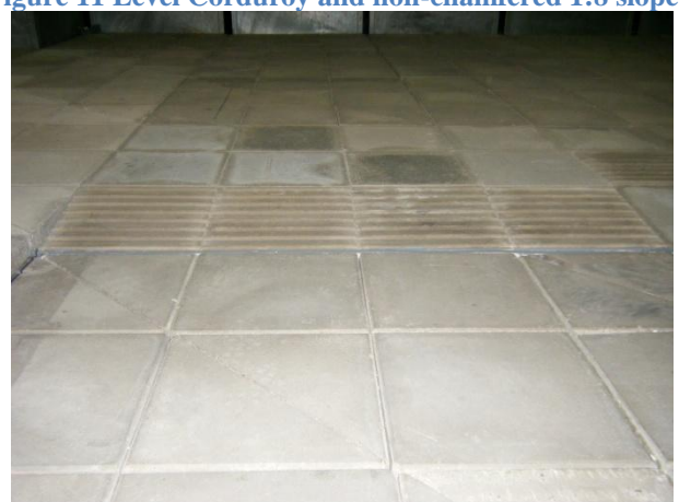
Figure 13 Corduroy Hazard Warning on 1:8 slope
