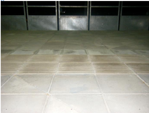
Figure 10 Corduroy Hazard Warning
