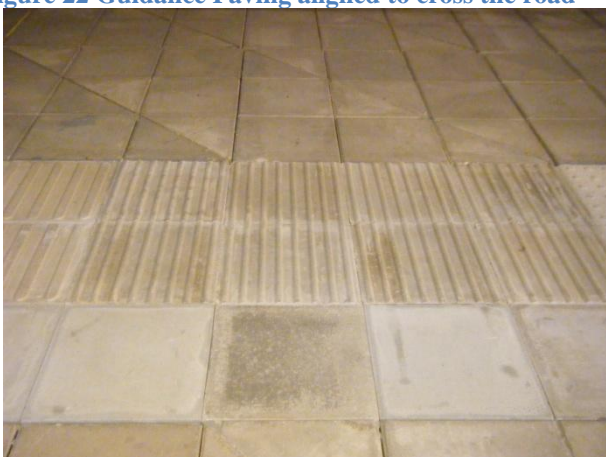
Figure 24 Corduroy Hazard Warning aligned to cross the road
