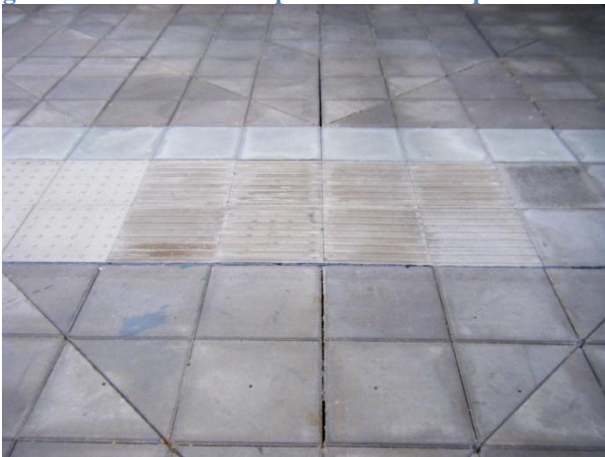
Figure 16 Corduroy Hazard Warning at 1:24 slope
